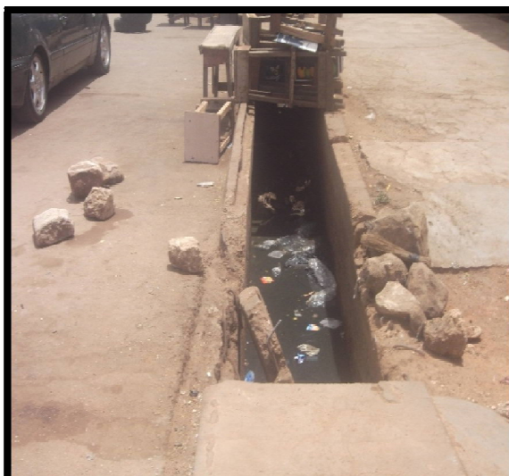
Figure 12: Broken Drainage with Stagnant Dirt Water Source: Researchers' Field Survey, 2019
