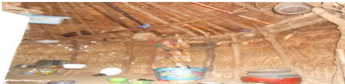
Figure 5: Internal appearance of the conical roof. Source: Adekeye, O. F: ( google scholar.com/scholar )
